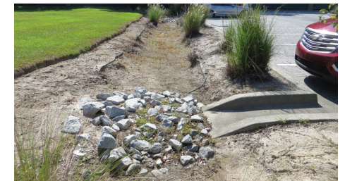
8 PRETREATMENT EROSION (FILTER STRIPS), 14 MULCH (NONE), & 24 PLANT DENSITY (POOR)
