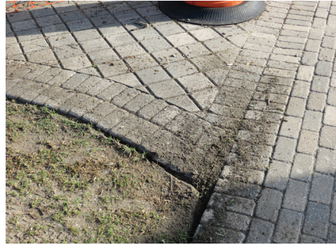
5 UNSTABLE DRAINAGE AREA
