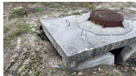
19 OUTLET STRUCTURE EROSION
