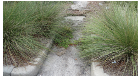
5 INLET STRUCTURE DEBRIS & SEDIMENT
