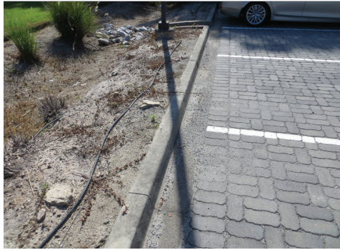
5 UNSTABLE DRAINAGE AREA
