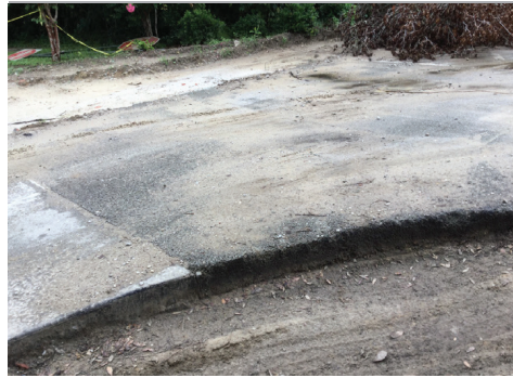
5 UNSTABLE DRAINAGE AREA & 13 SEDIMENT (POOR)
