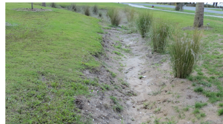
8 INLET EROSION (GRASS CHANNEL)
