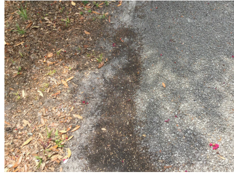
5 UNSTABLE DRAINAGE AREA & 14 DEBRIS (MARGINAL)
