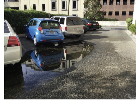
6 PONDING / STANDING WATER
