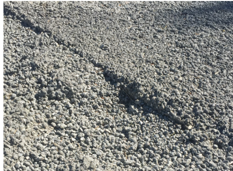
7 CRACKING & 15 RAVELING (POOR)
