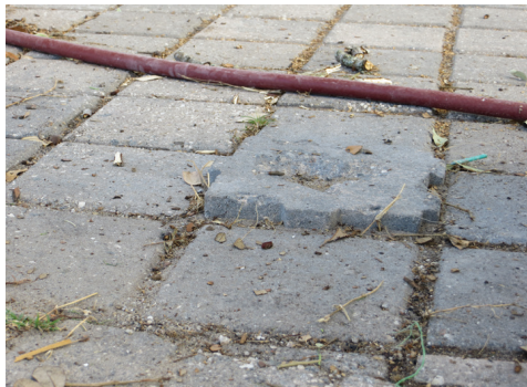
8 STRUCTURAL & 15 SEDIMENT (POOR)
