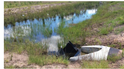
16 Lack of Vegetation & Embankment Erosion
