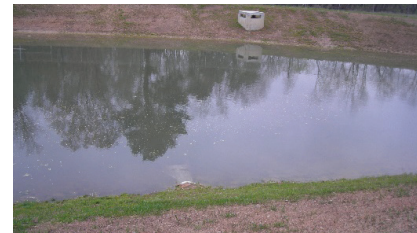
16 Lack of Vegetation
