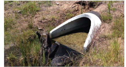
4 Slope & Pipe Erosion
