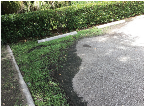
6 STANDING WATER, 12 VEGETATION (POOR) & 13 SEDIMENT (POOR)
