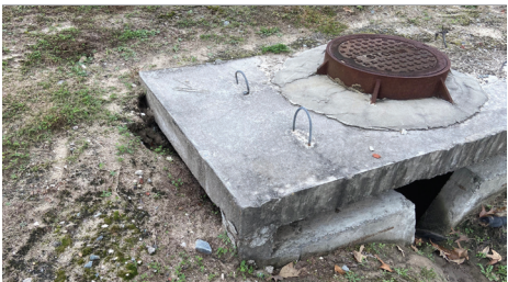
19 OUTLET STRUCTURE EROSION
