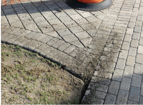
5 UNSTABLE DRAINAGE AREA
