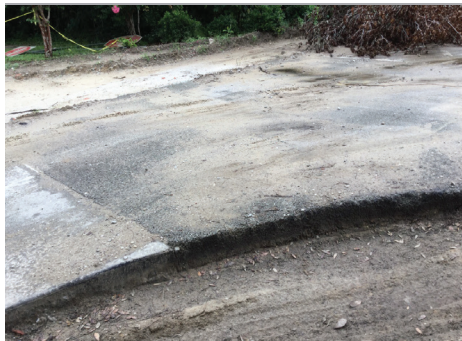
5 UNSTABLE DRAINAGE AREA & 13 SEDIMENT (POOR)
