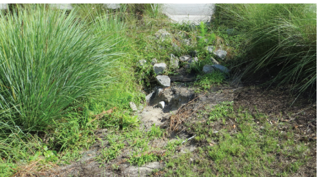
8 INLET EROSION (ROCK PLUNGE POOL)
