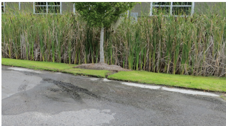
11 EXCESSIVE PONDING (CATTAILS & STAINING)
