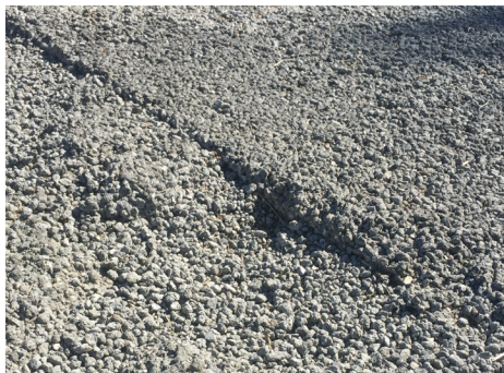
7 CRACKING & 15 RAVELING (POOR)
