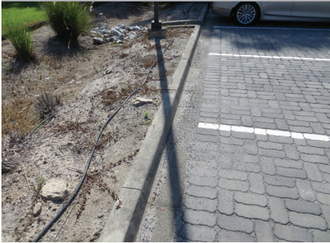
5 UNSTABLE DRAINAGE AREA
