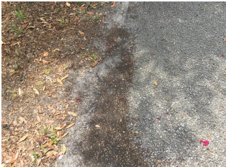
5 UNSTABLE DRAINAGE AREA & 14 DEBRIS (MARGINAL)
