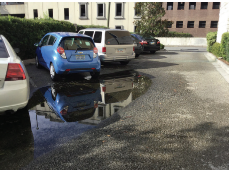
6 PONDING / STANDING WATER
