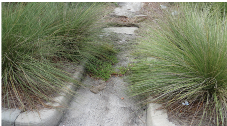
5 INLET STRUCTURE DEBRIS & SEDIMENT
